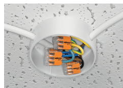
Lighting distribution in a ceiling canopy
