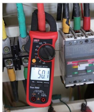
High voltage (600V) frequency measurement
